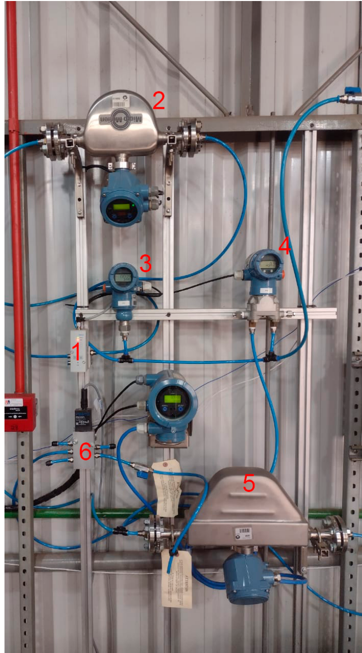
Figure 4.2 – Sensors installed on the gas line.
