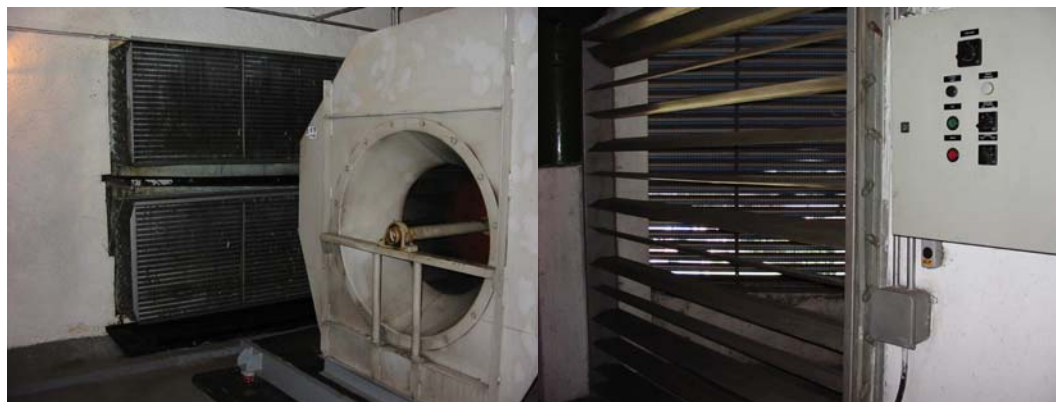
Figura 5.6.2.2 – Fancoil e damper
